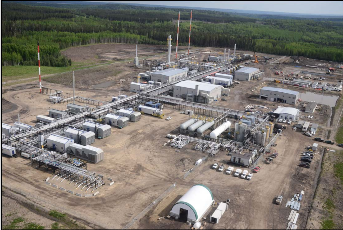
Paramount's 8-13 Musreau Complex: 45 MMcf/d Refrigeration Facility (foreground) & 200 MMcf/d Deep Cut Facility (background)
